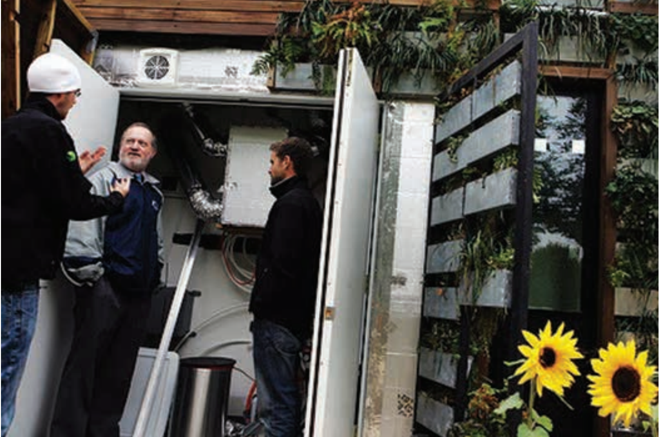
All of Natural Fusion's building systems are centralized in a common mechanical space called the "Nexus"
