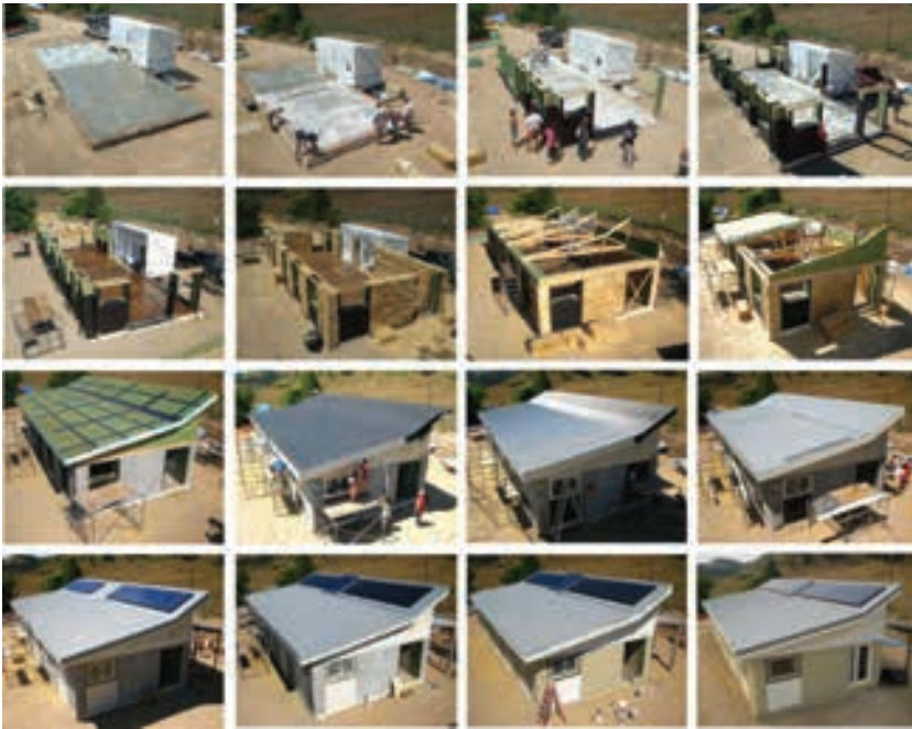
Fig.3: Time-lapse construction sequence of MorningStar MT. The Utility Core was prefabricated, transported to the site, and set on a prepared foundation. The home's living space was site-constructed by volunteer labor using straw-bale construction for exterior walls and structurally insulated panels for the roof. A solar-electric array and evacuated-tube solar thermal panels were installed on the south-facing roof, providing heat, hot water and power to the home. (Courtesy of the 2007 Penn State Solar Decathlon Team and the Penn State Center for Sustainability American Indian Housing Initiative)
