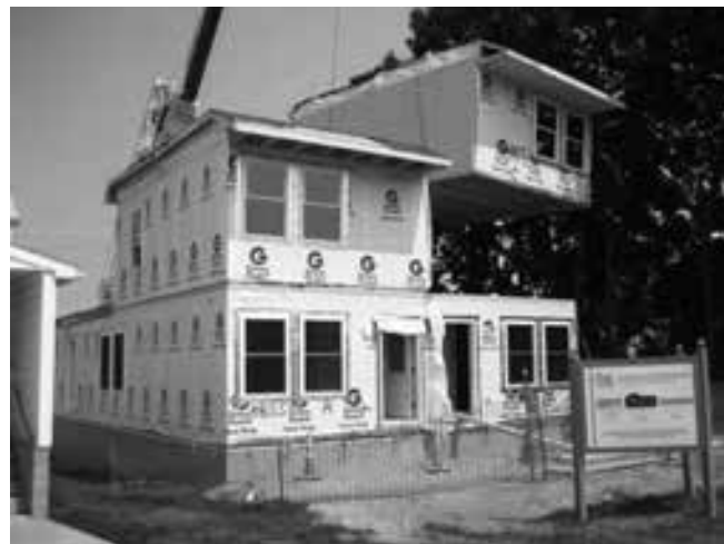
Fig. 9: Modules of the EEHP duplex being set on site. (Photograph by author)
