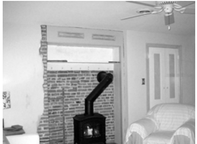
Fig. 7: Efficient stove supplementing hot water heating system in “Pod”.
